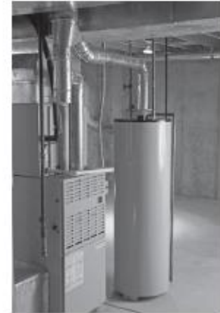
Heating systems (© Comstock RF.)
